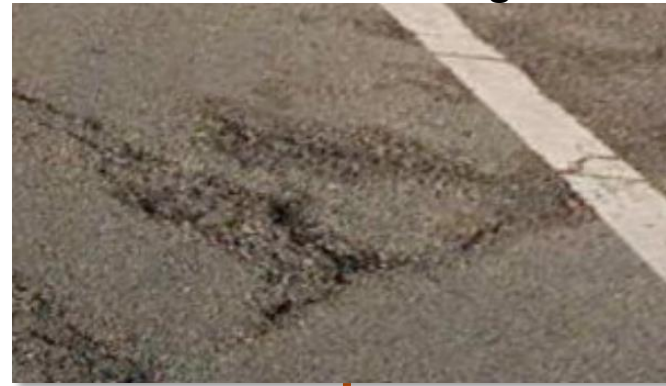
Defect in normal image
